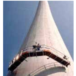
Chimney Access - E. Thomson Denmark
