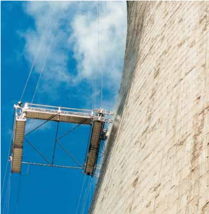
Cooling Tower - Poland
